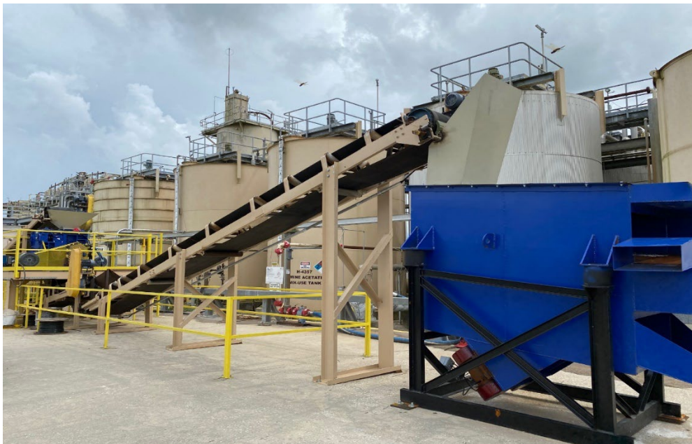
Crushing and Screening System for Pilot PCJ Pilot PCJ Control Room
